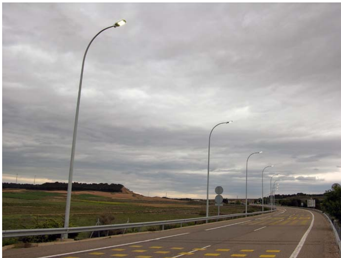
LED Street Lights in Bilbao, Spain
